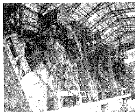
Low Pressure Extraction System
