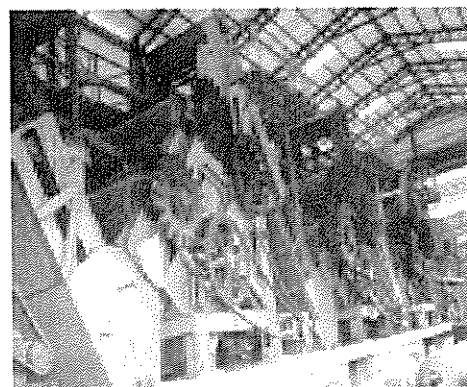
Low Pressure Extraction System
